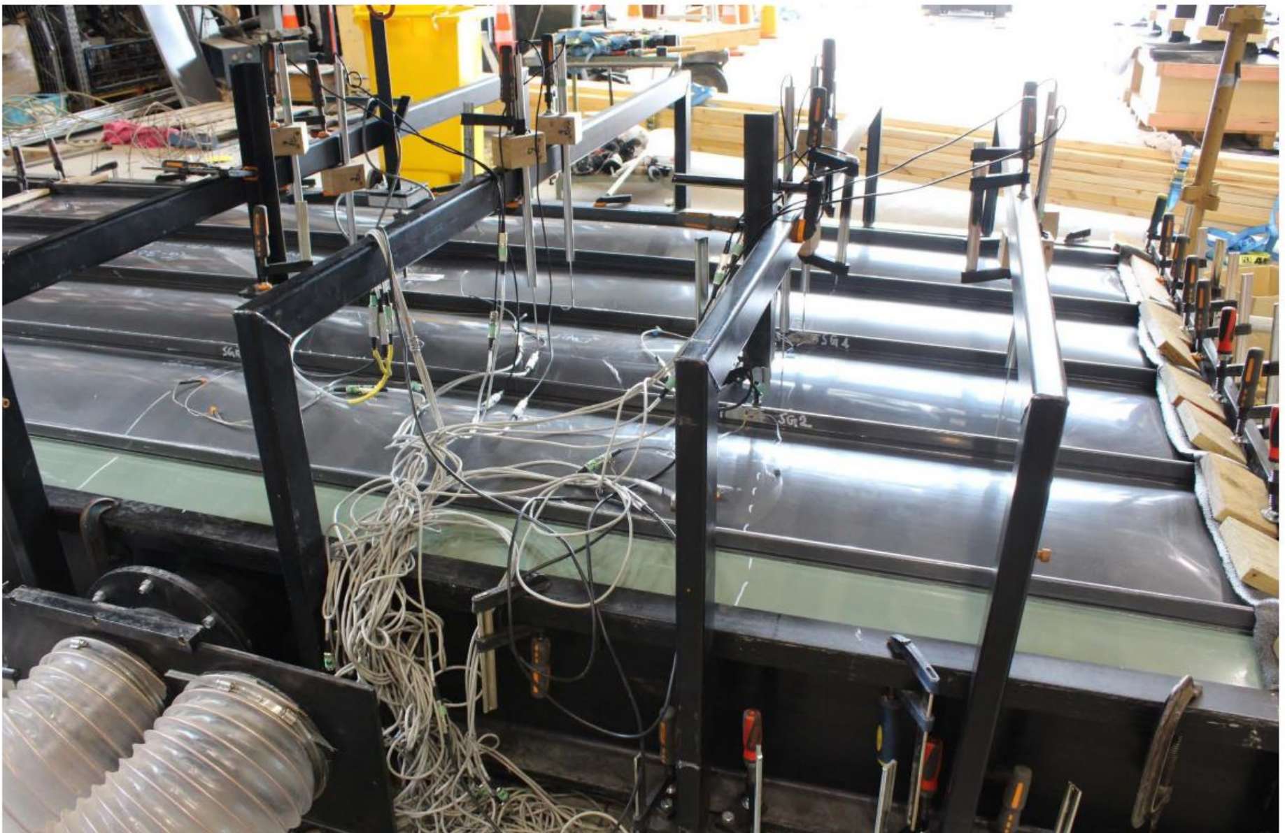
Fig. 6: Super seam cladding of 450 mm pan width in static uplift test for “Superseam-S2000-t0.55” at the middle of the test (end of tests)
